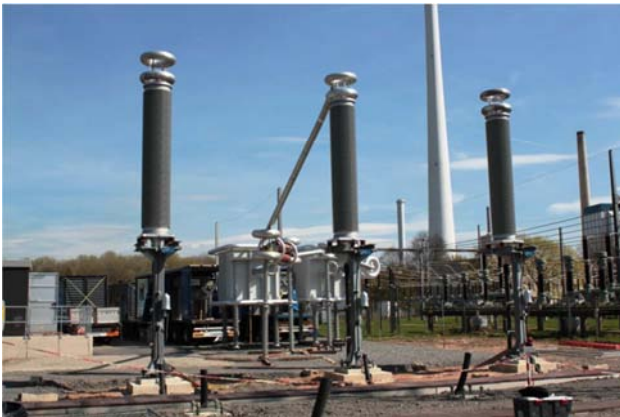
Figure 6: Resonant test equipment for 374 kV
