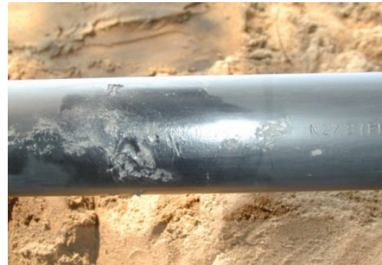
Fig. 1: Cable sheath after a dielectric breakdown
