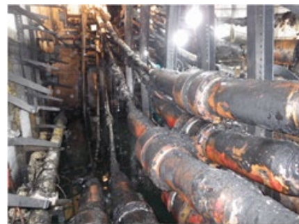
Fig. 1 Site of 2016 tunnel fire
