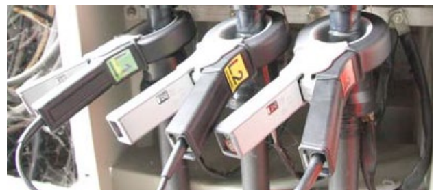
Fig. 1: Inductors placed on screen grounding cables
