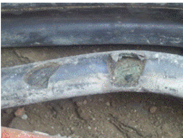
Fig. 1: Damaged 138 kV XLPE cable.
