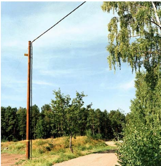
Fig.1. Cable from coming up from ground and going further as aerial cable
