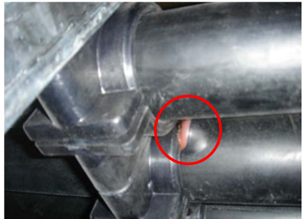
Fig. 1: Example of bubbling/melting of outer sheath under cable cleat caused by heat from laminate and screen wires [1].
