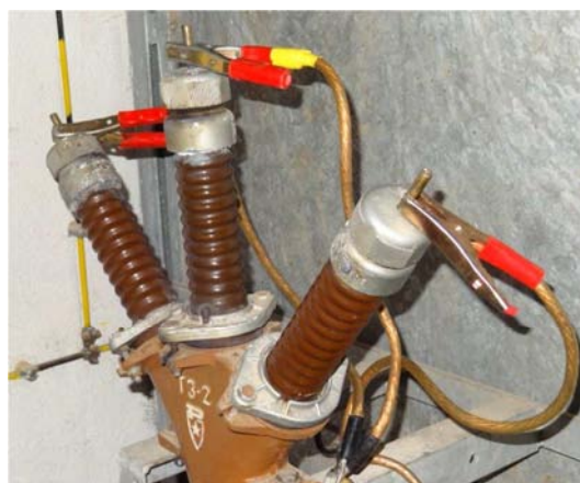
Fig.1: old 3-phase termination of a 3-lead cable
