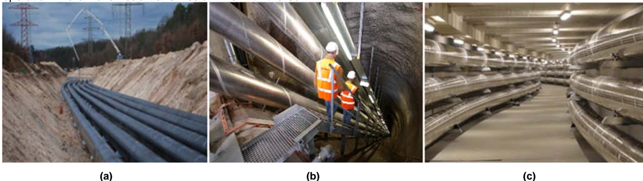
Fig. 2: Installation of GIL: (a) Directly-buried; (b) inclined tunnel; (c) tunnel with bending radius
