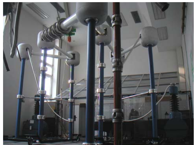
Figure 1: Photo of the experimental VLF test voltage source at the TU-Berlin
