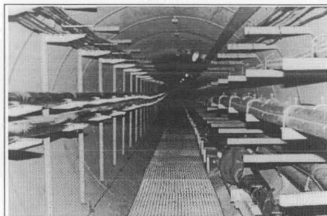
Figure 1. Tunnel containing 220kV power (with a joint at bottom right hand side), communication and service cables.
