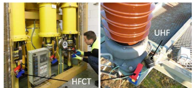
Figure 1. Sensors installation at the GIS and OHL cable terminations
