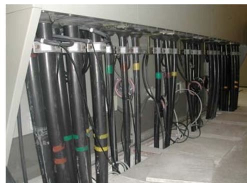
Fig. 2: Current sensors on cables
