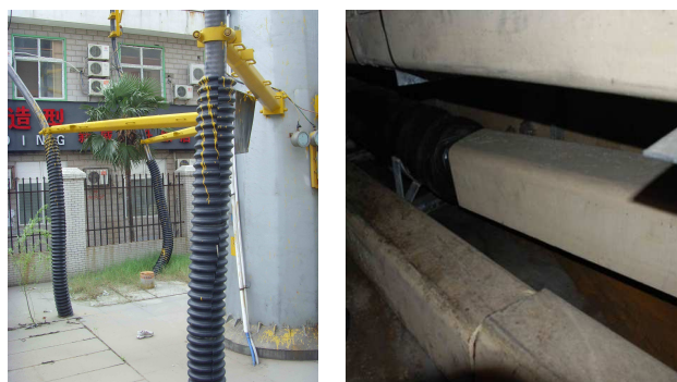
(a) Cable in vertical protect tube (b) Single cable in fire-proof box
