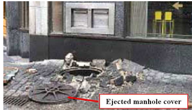
Fig. 1: Explosion in an underground vault
