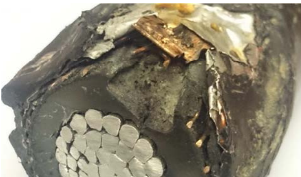
Fig. 4: Detailed damage from installation in Fig. 3.
