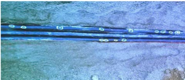
Fig. 3: Multiple damages in power cable sheath close to end termination. Laminate and copper screen not connected.
