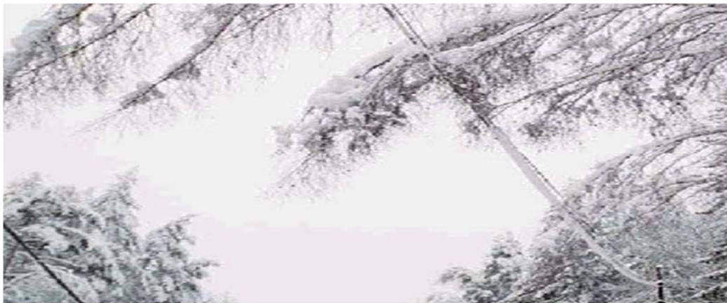
Fig 1 Snow covered heavy branches on live cable
