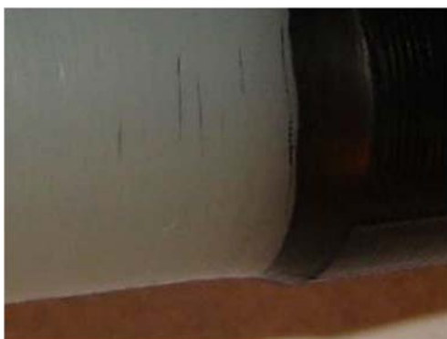
Figure 1: Found defect in 20kV joint
