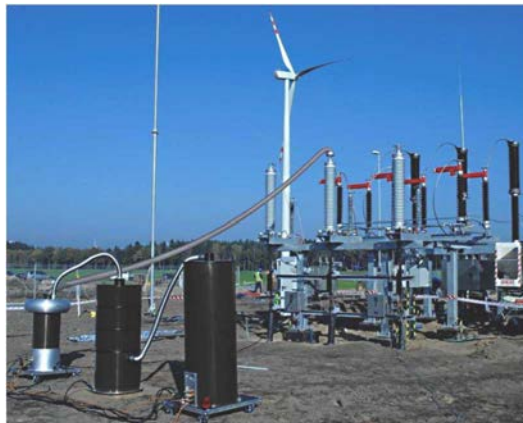
Figure 1: Example of a DAC after-laying test of a 6.4 km long 110kV XLPE cable circuit.
