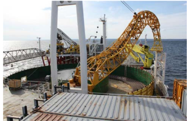
Figure 7: example of export XLPE cable installation.
