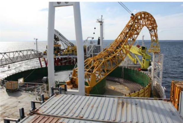
Figure 7 shows an example of export XLPE cable installation.
