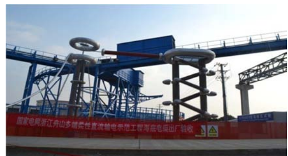
Fig.9 DC voltage test equipment
