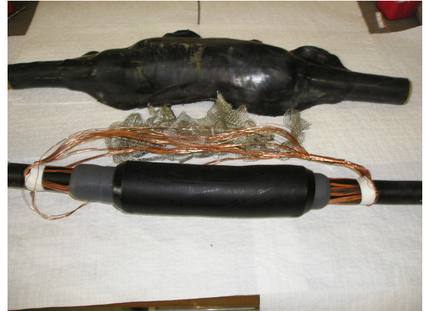
Figure 7: Splice body not correctly positioned
