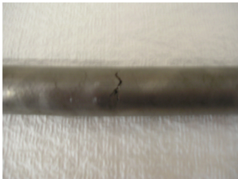
Figure 6: investigation results: Cracks in the lead sheath
