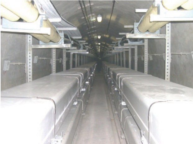
Figure 2: A typical installation of the underground 154 kV power cables at S district, Seoul, Korea
