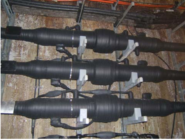
Figure 1: A typical installation of the underground 154 kV power cables at S district ,Seoul, Korea
