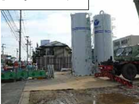
Silo (pouring of materials)
