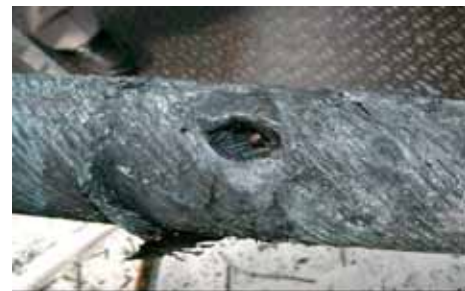
Figure 2: Cable breakdown in a tunnel duct
