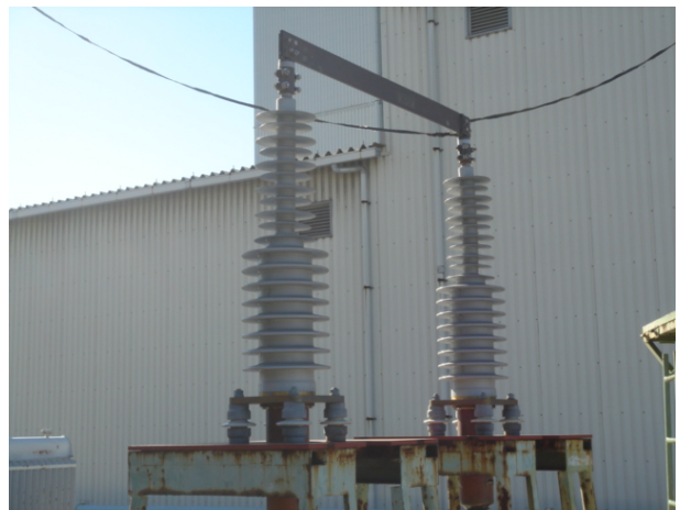
Figure.6 View of dry-type out-door terminations in long-term tests
