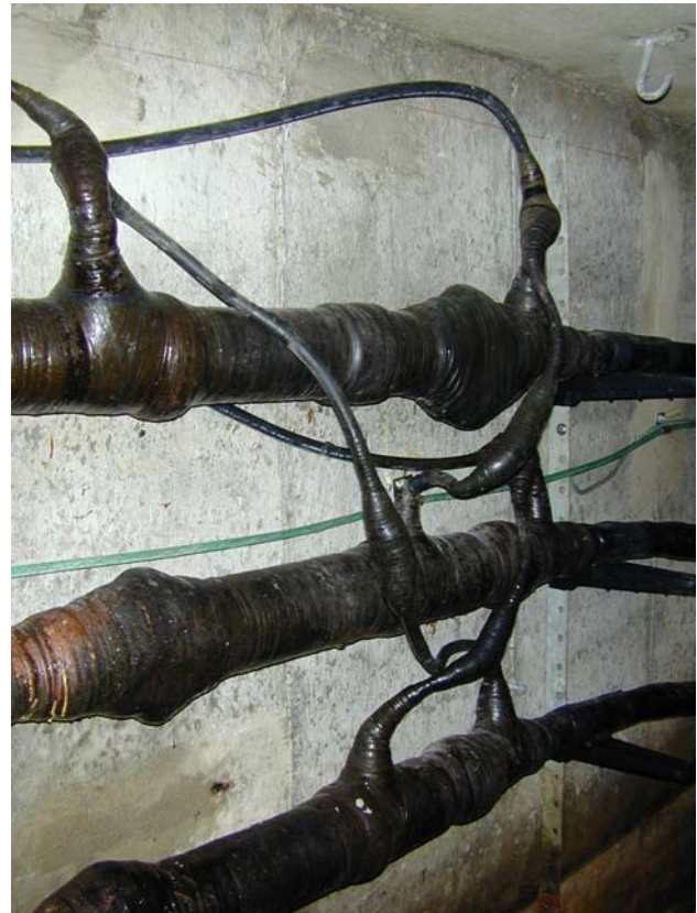
Figure 3. 120kV sectionalized joints in a manhole
