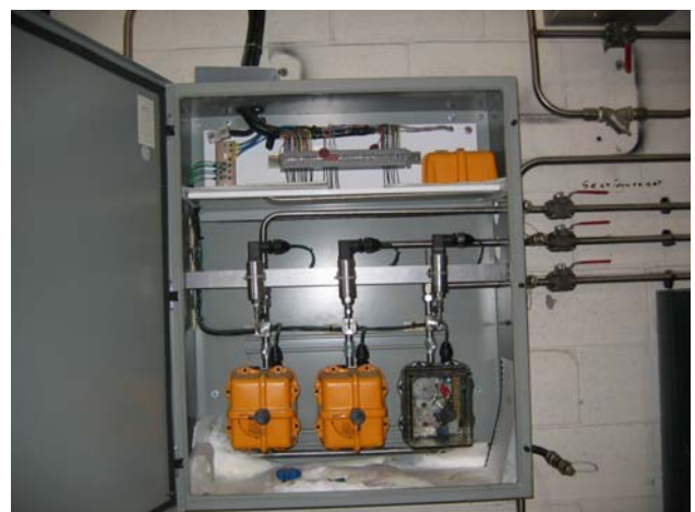
Figure 4. Automated oil pressure monitoring system.
