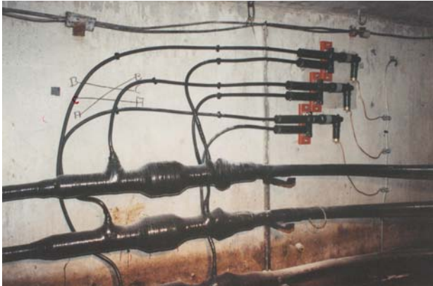
Figure 5. Cross bonding system in a manhole.
