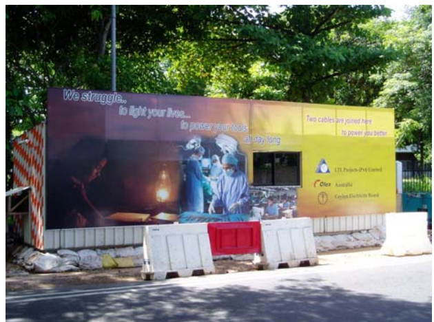
Photo 8: Specially designed enclosure over joint bay for HV cable jointing in controlled environment.
