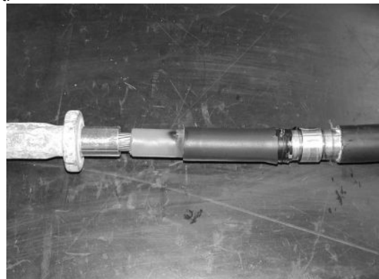
Figure 15: Appearance of the inside of the termination
