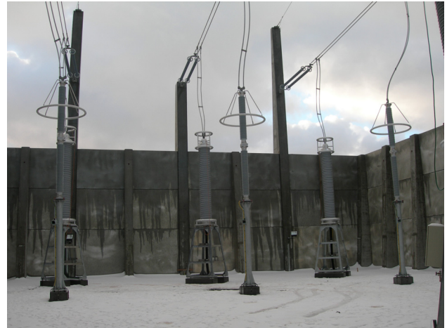
Figure 5. Outdoor terminations at Hamneset.
