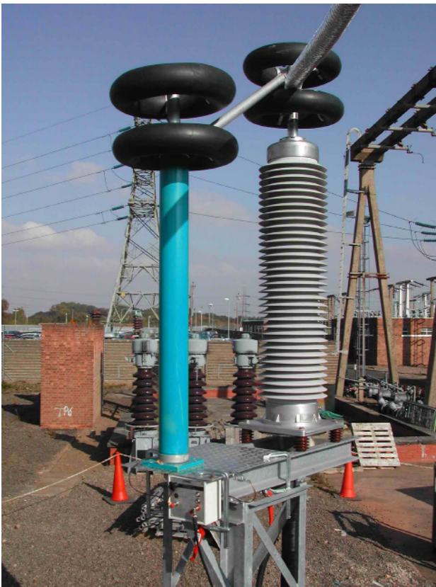
Figure 1 Coupling capacitor next to termination
