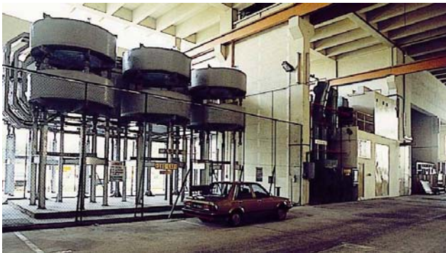
Figure 13: 230 kV, 0-100 Mvar TCR
