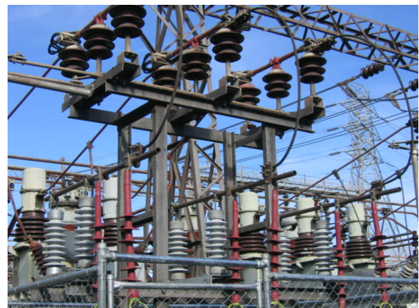
Figure 2. 33kV Feeder cable terminations
