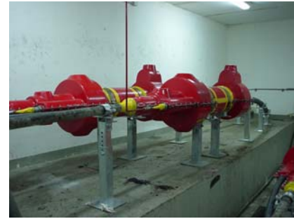
Figure 7: Oil-XLPE cable transition joint
