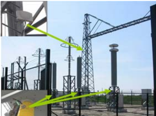
Figure 3: Overview of one side of a 380 kV cable system. The top inset shows the antenna which is used to make the wireless communication with the main computer and other measuring units possible. The lower inset shows a detail of the internal inductive PD sensor.
