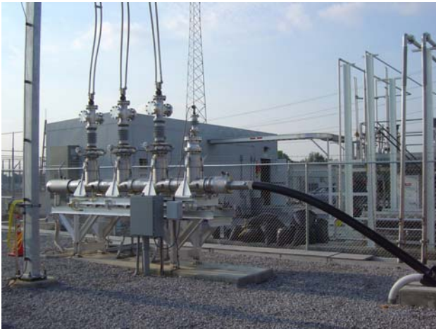
Figure 4: Triax HTS cable termination.
