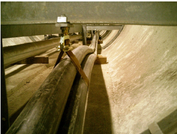
Figure 6: Cables hanging in "waves" below steel girders in the tunnel.
