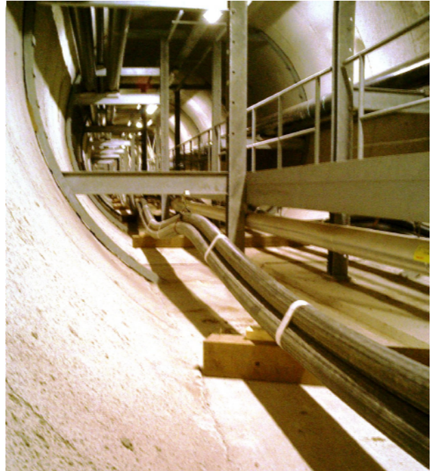
Figure 1: An orderly multi-purpose tunnel interior with HV cables and different pipes for transporting liquids and gasses.
