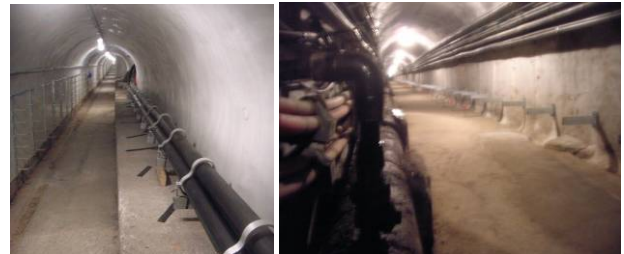
Figure 12: Cables in shared services galleries
