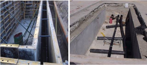
Figure 9: old joint bay
