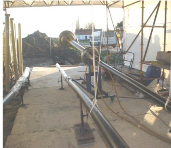
Figure 2: temporary termination used for testing the link in three sub-links (injection of 2U_0 )
