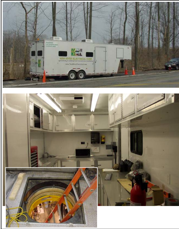
Figure 7: Outer and inner views of the trailer with the integrated access to the manhole
