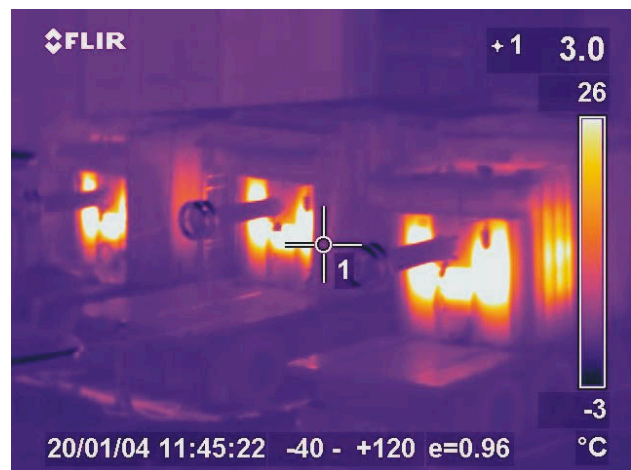
Fig.7 Test of the AC test system (280kV test voltage /1h)
