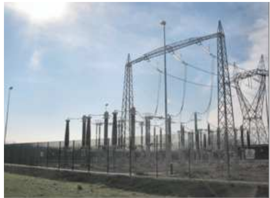
Figure 7: Turbigo-Rho transition station
