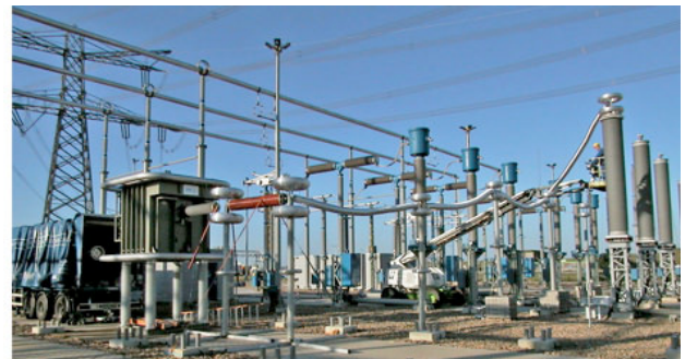
Figure 6: 380 kV test set-up in a substation
