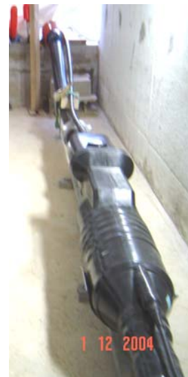
Figure 4 : Cross bonding joint with embedded capacitive PD sensor
