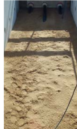
Figure 13 : Joint bay filled with sand saturated with salted water
