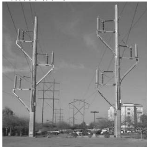
Figure 6: 150 kV terminations with composite insulator installed on an OHL- UGC transition pole.
