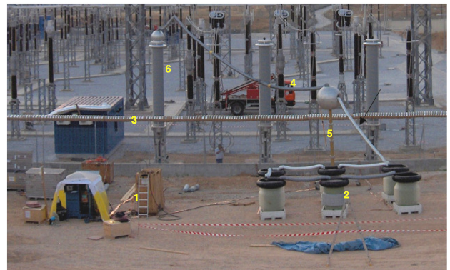
figure 5: set-up during commissioning test
