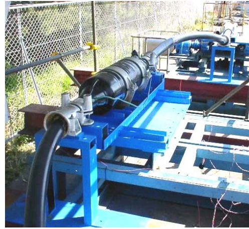
Fig. 18 View of 154 kV-class CSJ Subjected to Load Cycling and Thermo-mechanical Tests
