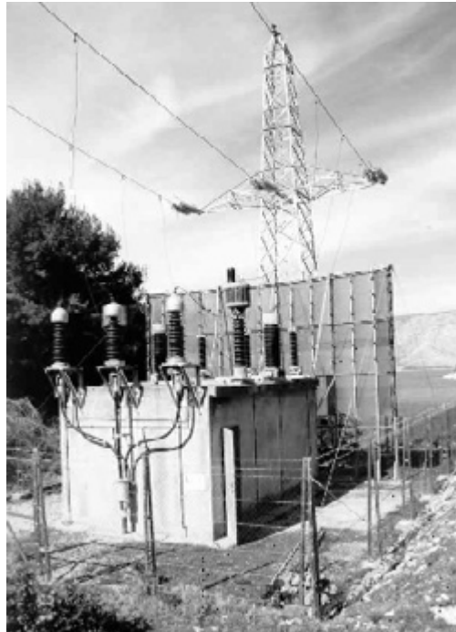
Fig. 3. Travna Cable Station – A net structure for protection from the sea salt sediment
